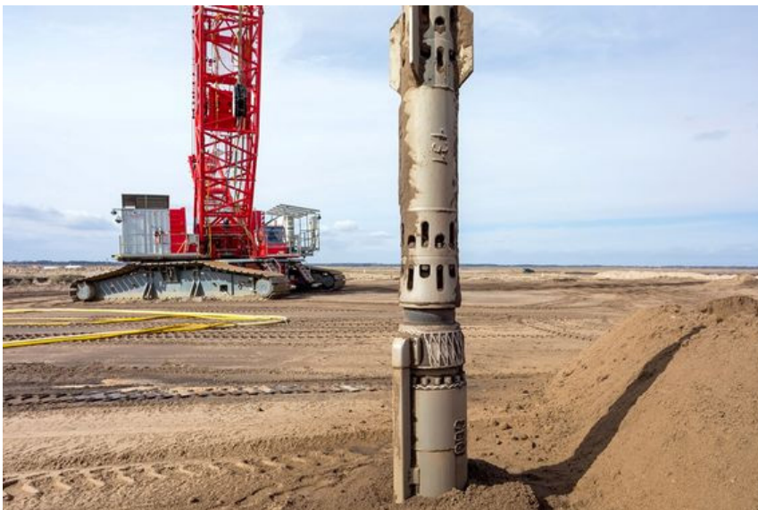
Figure 4.5: Deep vibratory compaction in action in test field at Cottbus, Germany (GMB GmbH, 2017b)
