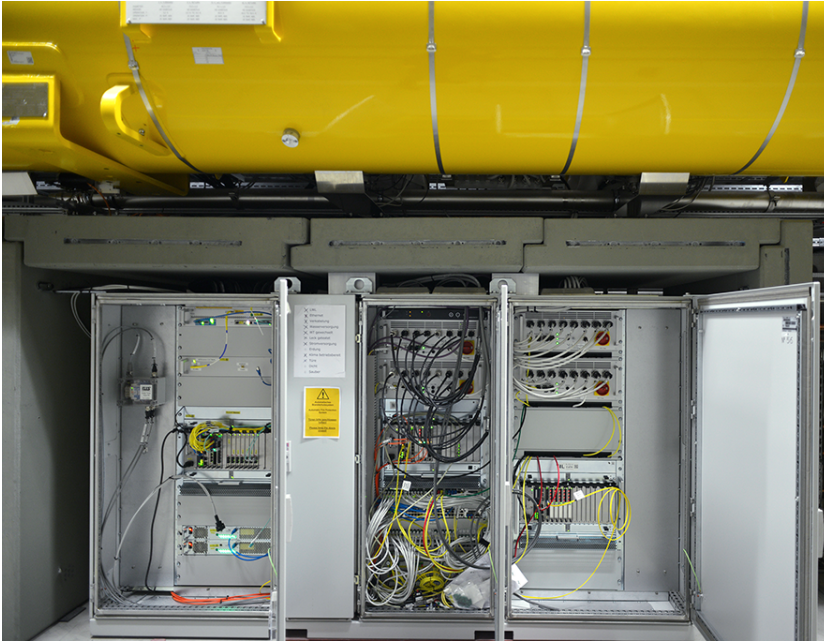
FIGURE 2.2: Picture of the physical setup of the cabinets under the cryomodules inside the European XFEL accelerator tunnel. The left cabinet contains the LLRF system.
