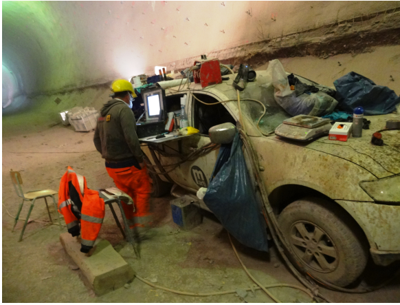
Figure 7.9: The injection unit “Mob. PU” is mounted directly to a pick-up truck. Foreman and equipment are directly exposed to the tunnel.
