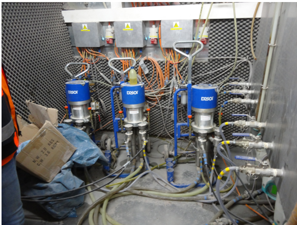
Figure 7.11: Three pumps installed in an AC injection unit.
