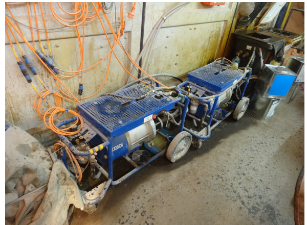
Figure 7.12: Two pumps installed in a PU injection unit.
