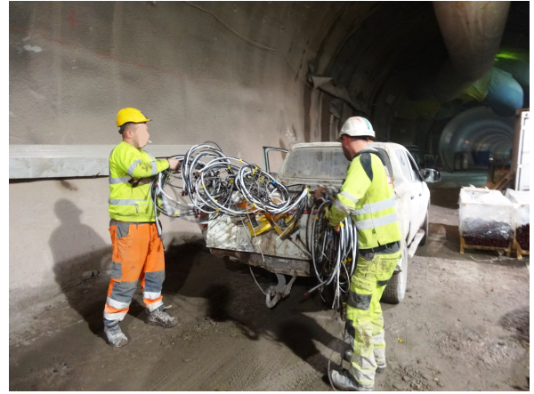
Figure 7.10: Workers of the maintenance team unload injection heads, packer and hoses for further cleaning from the transport pick-up truck.
