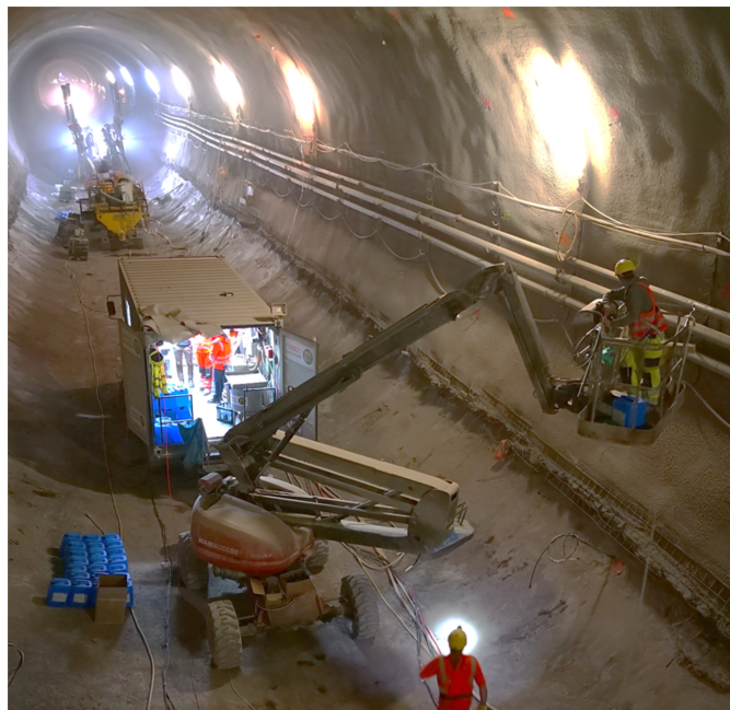
Figure 5.12: Production System. Depicted are the drilling unit (top, left), the truck mounted GEA container (middle) and a lifting platform (bottom). Blue canisters contain a chemical component for the grouting agent. Boreholes in the tunnel wall have been marked with colored spray paint.
