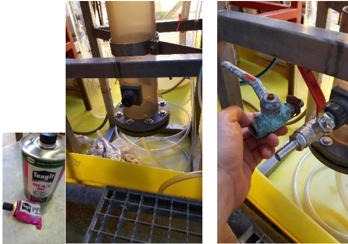
Figure 57. Conditioning of SFBBR-2. Left: Sealing of leakage with glue Tangit & PVC cleaner; Right: Replacement of downwash line valve
