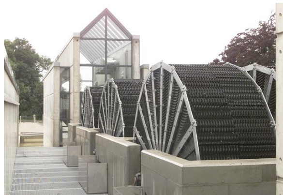
Figure 27. RBC system (Balteau, 2012)
