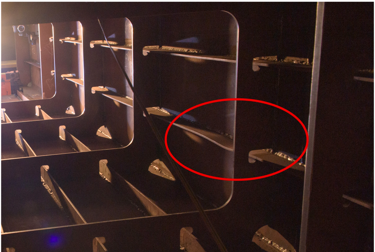
Fig. 14. Large initial deflections of the stiffener before test.
