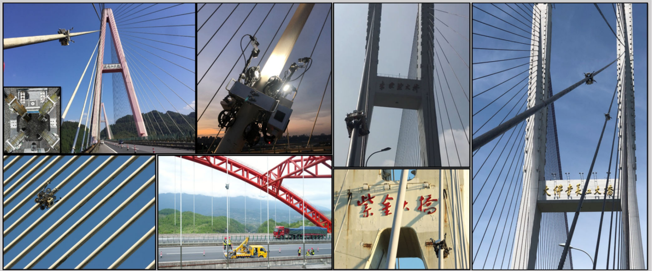
FIGURE 19 | Field test and realistic deployment of the climbing platform, which has been tested on more than 500 stay cables, with an accumulative trip of approximately half a million meters. [Color figure can be viewed at wileyonlinelibrary.com ]
