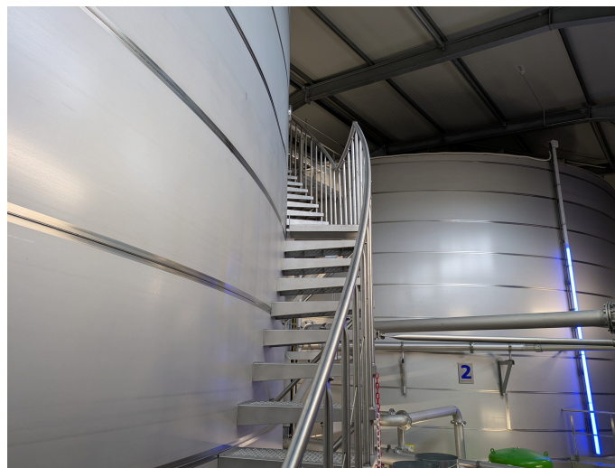
Figure 21 – Two-tank system for water storage at the water supply and treatment center (Versorgungsbetriebe Helgoland) at Helgoland, Germany.
