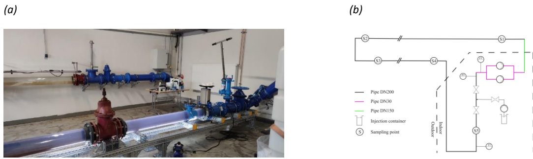
Figure 4: Picture (a) from the indoor part and total flow chart sketch (b) of the Hamburg Wasser pilot plant.
