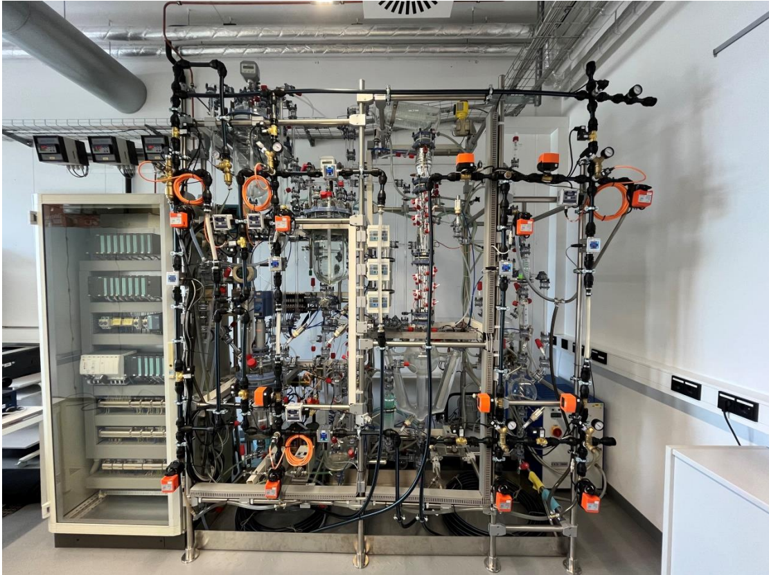
Figure 15: TU Ilmenau testbed.
