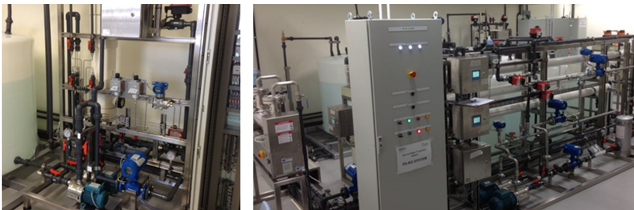
Figure 2.7: Physical process infrastructure and field equipment [155]
