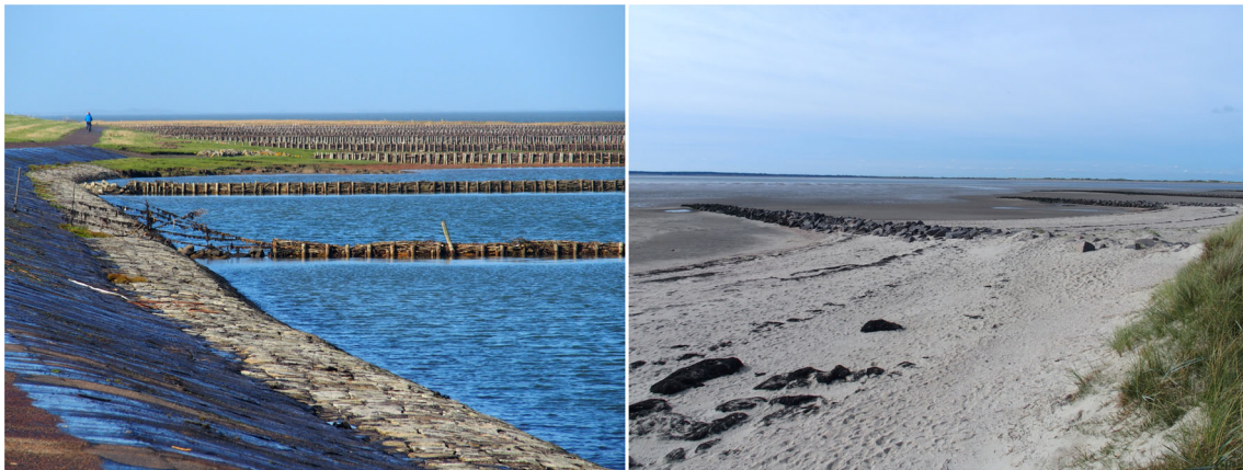
Fig. 11 Dike with adjacent fields of brushwood groynes in the north-east of Föhr with already developed foreland in the back (left) and beach with rubble stone groynes in front of the Clinic Utersum (right), Photos: P. Jordan
